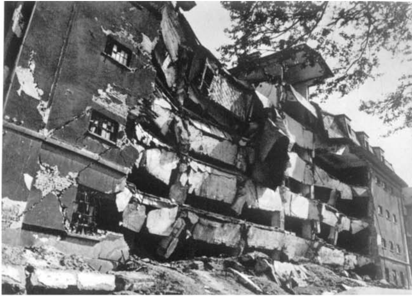
Fig. 6. Pancake failure of tobacco factory masonry building in central part of Skopje
