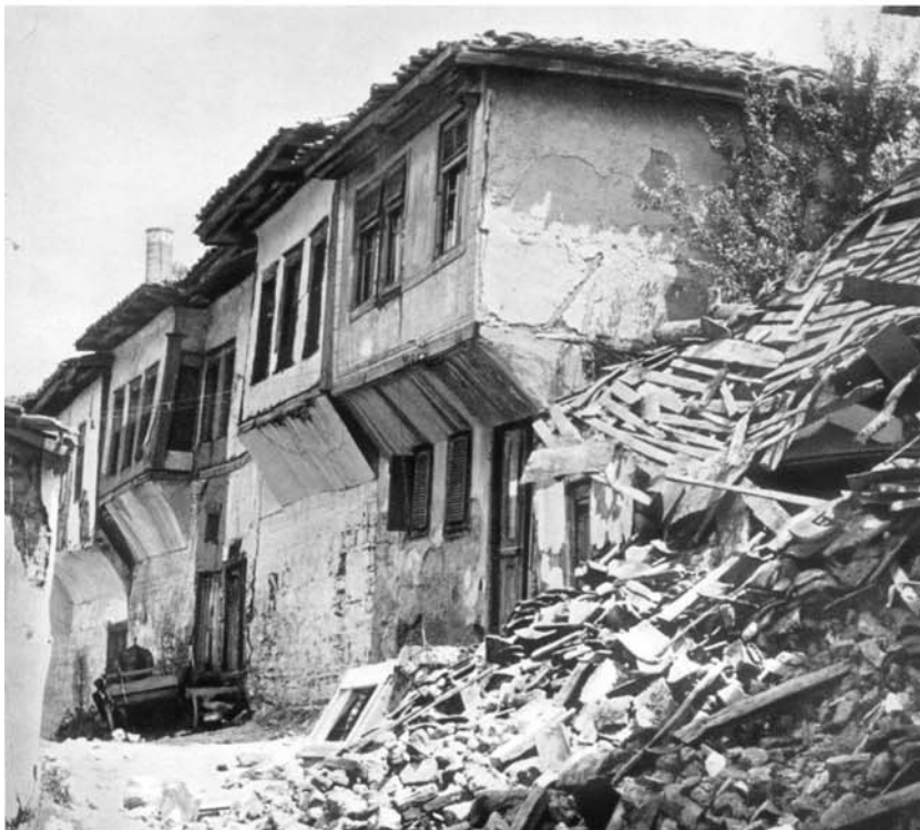
Fig. 7. Slight damage of wood-framed Macedonian dwelling (left) and failure of rubble stone masonry dwelling (right) in the central part of Skopje
