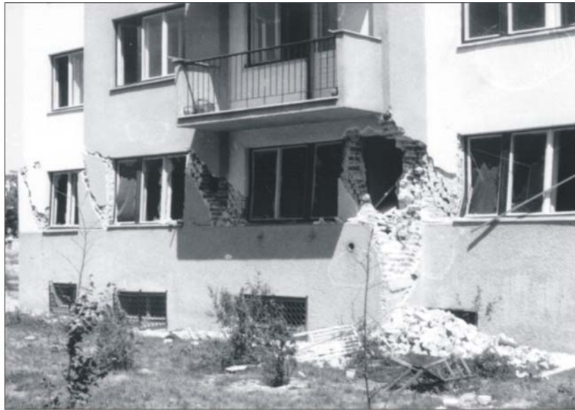
Fig. 4. Damage pattern of five storey masonry buildings of Type B
