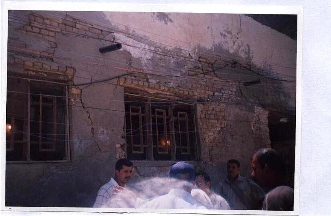
Fig 5 AL-refaae: diagonal and horizontal Cracks from the basement to the roofs .
