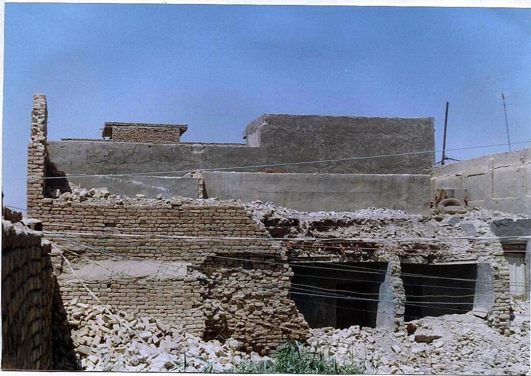
Fig.1 AL-refaee: total destruction of the main wall and the roof of the house.
